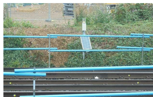
The track monitoring devices will measure track movement during the main construction works. They have been installed on the rails and are fitted with solar powered transmitters. The transmitters send data to a computer. This modern system eliminates the need for manual surveying as well as potential risks
