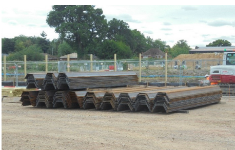
The sheet piling will support the existing ground along the railway during the new bridge construction
