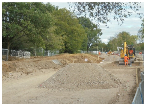
The new road is beginning to take shape. The ground, seen here, was stripped from top-soil ready for the new road foundation
