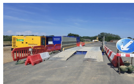
With daily movement of around 200 construction lorries, a new wheel wash system has been introduced to keep the roads clean of mud
