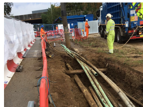
Vacuum excavation was carried out in the footways on Reading Road to safely reach buried services (water, gas, electrics, telecoms). These services required lowering underground and in some places were diverted entirely to accommodate the two new roundabouts
