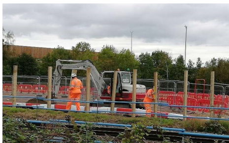
New swale cut through the site to allow for improved drainage of the road
