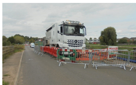
The first phase of construction works includes vacuum excavation for access to underground utilities (i.e. gas, electricity, telecoms)
