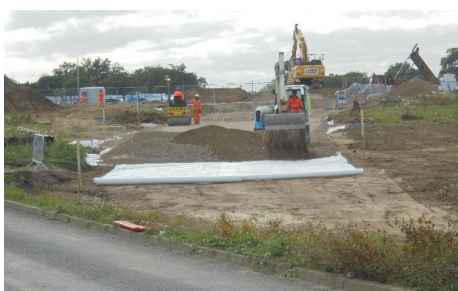
The first phase of works along Old Forest Road have so far included laying a top-soil strip and the installation of geotextile
