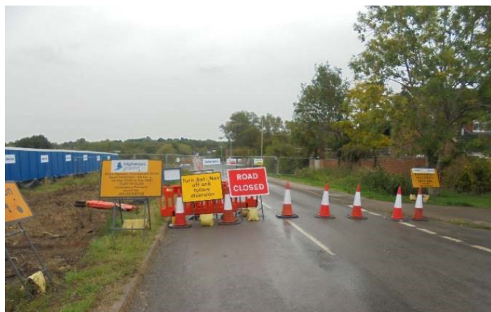
Section of Old Forest Road is now closed until March 2021. This is to allow us to construct a section of the new road which will connect to Toutley Road junction
