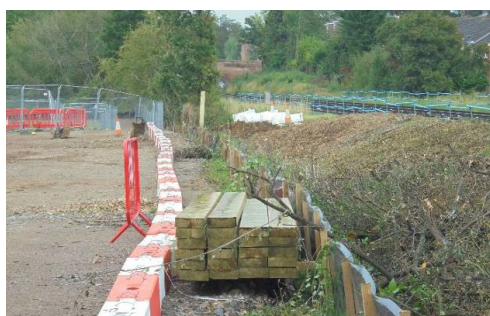
Red-white blocks linked together forming a barrier as a safety measure before timber hoarding is installed to prevent excavators and vehicles from encroaching into the railway boundary
