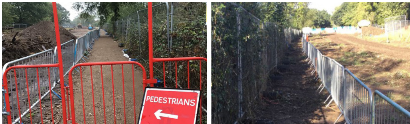
Winnersh Relief Road safety measure: A temporary pedestrian walkway has been installed through the northern roundabout site. This helps to create a visual exclusion zone between plant and pedestrian
