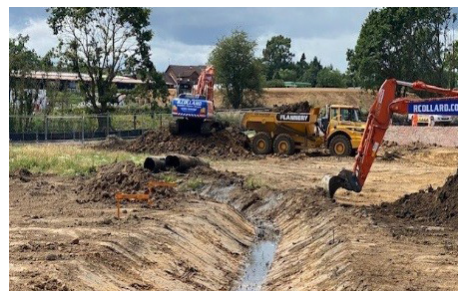
New swale cut through the site to allow for improved drainage of the road
