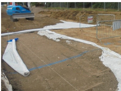
Geotextile material has been installed. This is a permeable fabric to help reinforce and protect the road as well as help the road to drain
