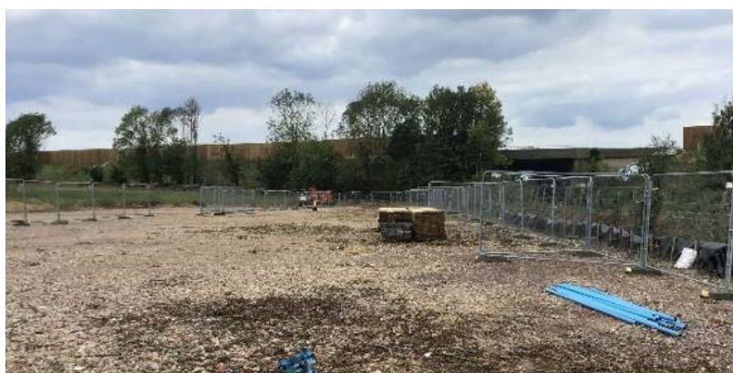
Special fencing and track monitoring devices have been installed on the rails along the train track to enable the earthworks in preparation for the new bridge over the railway
